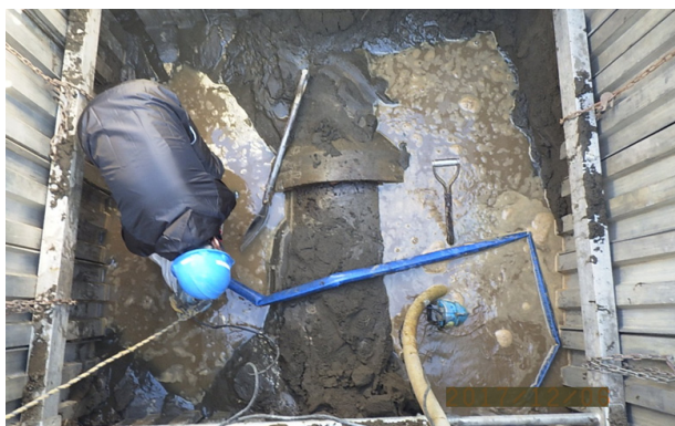
Figure 3: Sewer pipe and ground water (CASE-B)
